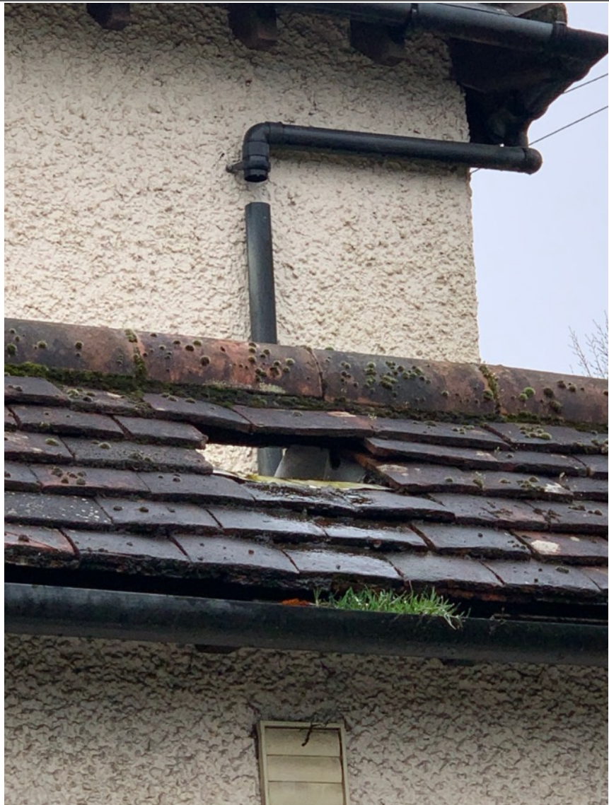
Photo showing loose vandalised downpipe. Note need to remove grass from gutter,
