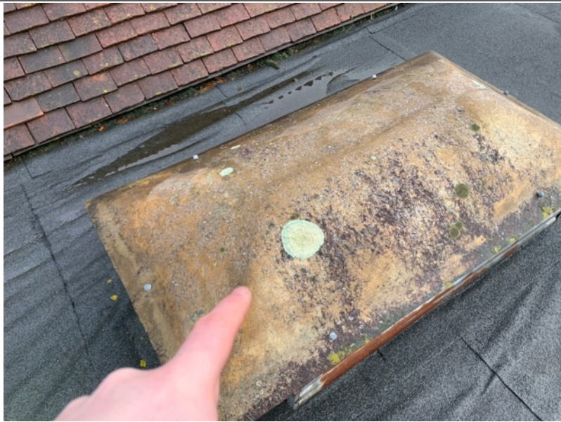
Photo showing polycarbonate roof dome in poor order
