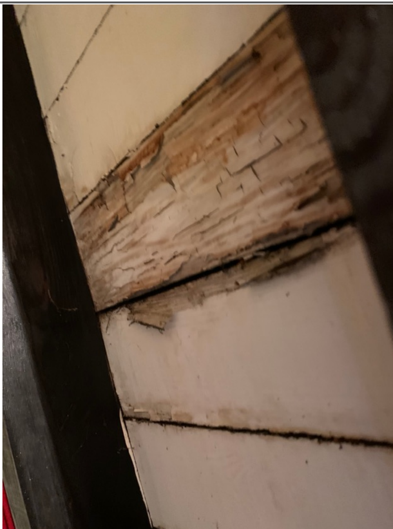
Photo showing decay of timber sarking board over the clerks office
