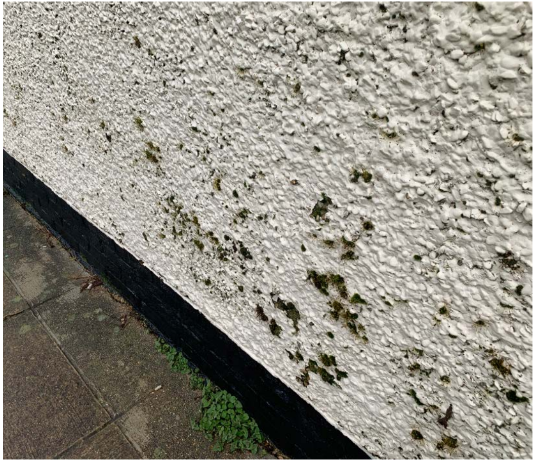
Photo showing porous render
