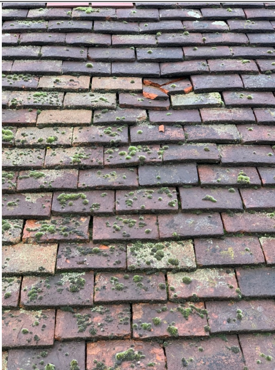
Photo showing impact damage to the roof
