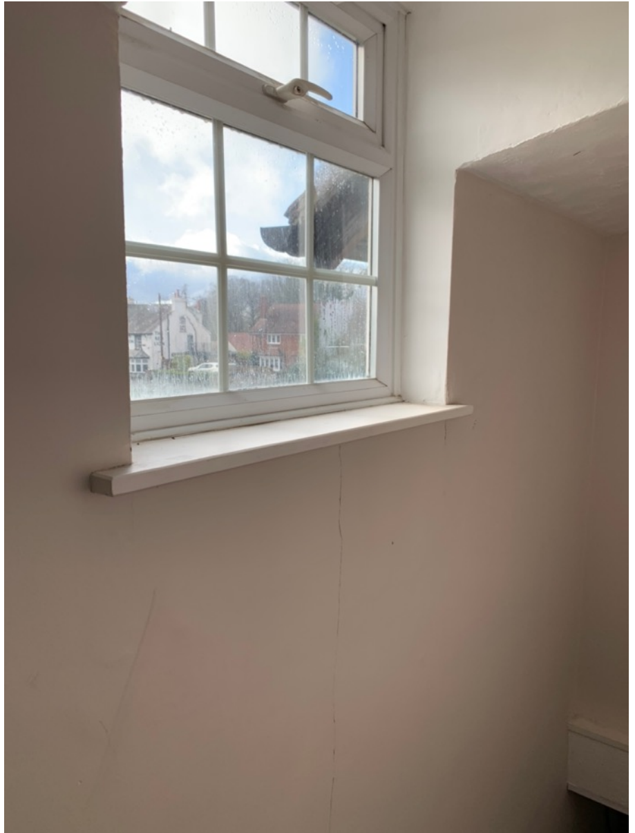
Photo showing condensation build up in glazed pane
