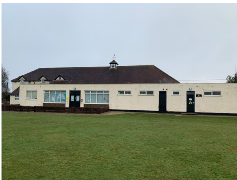
Photo showing rear single storey elevation with render in generally poor repair
