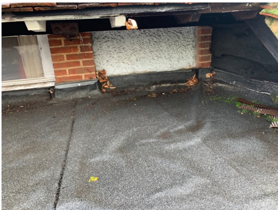
Photo Showing "bubbling" roofing felt .
