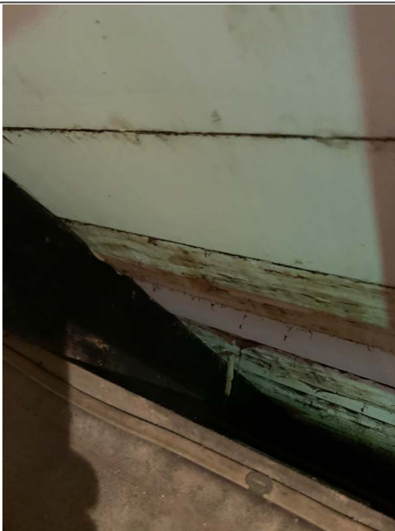
Photo showing signs of water ingress to the rear roof slope thought in line with external hole in the roof.
