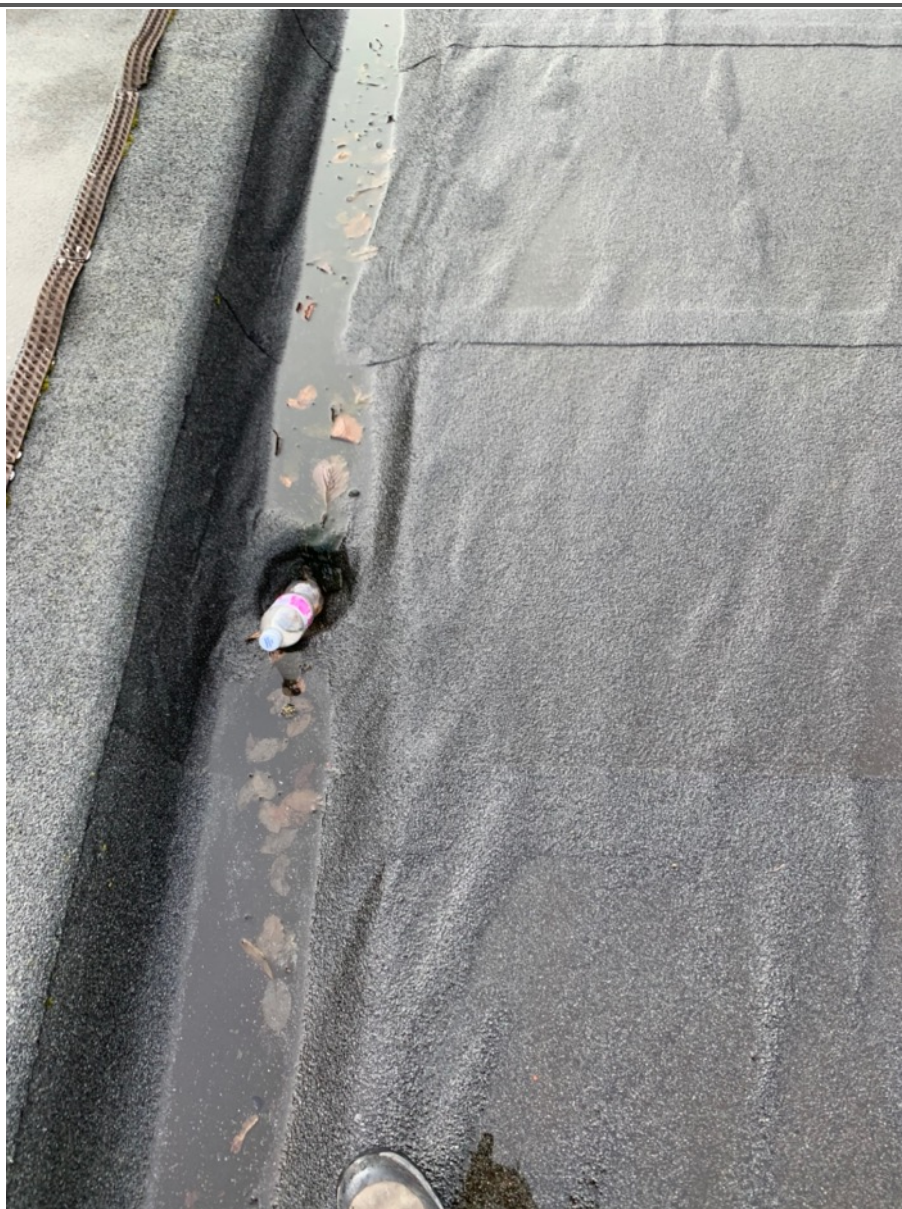
Photo of 1 of 3 bottles inserted into drainage gullies (thought vandalism)
