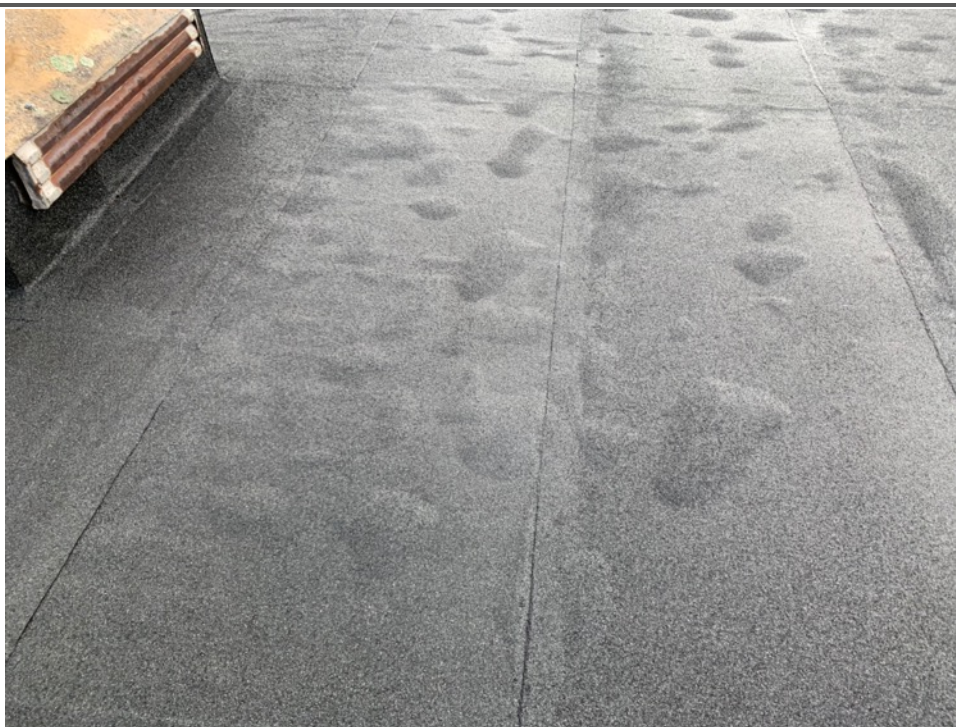
Photo Showing "bubbling" roofing felt .
