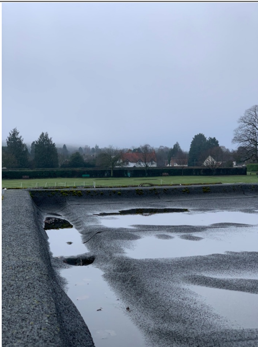
Photo showing ponding water around rainwater gulley indicating failure of water to flow away effectively
