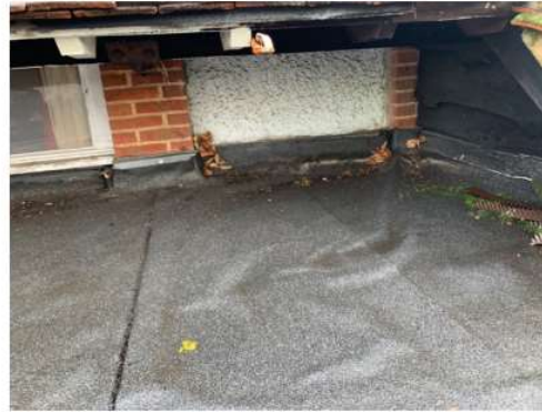
Photo Showing "bubbling" roofing felt .
