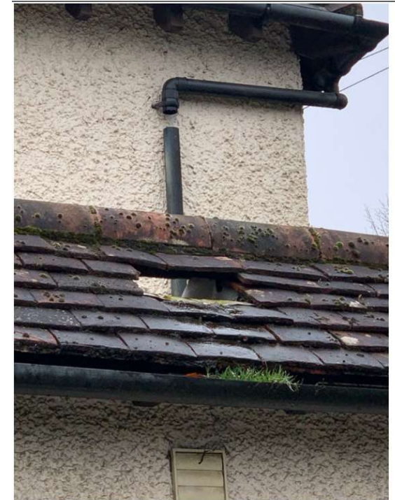
Photo showing loose vandalised downpipe. Note need to remove grass from gutter,
