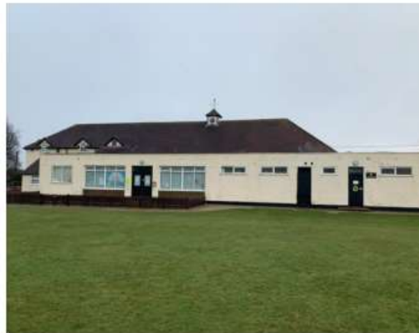
Photo showing rear single storey elevation with render in generally poor repair
