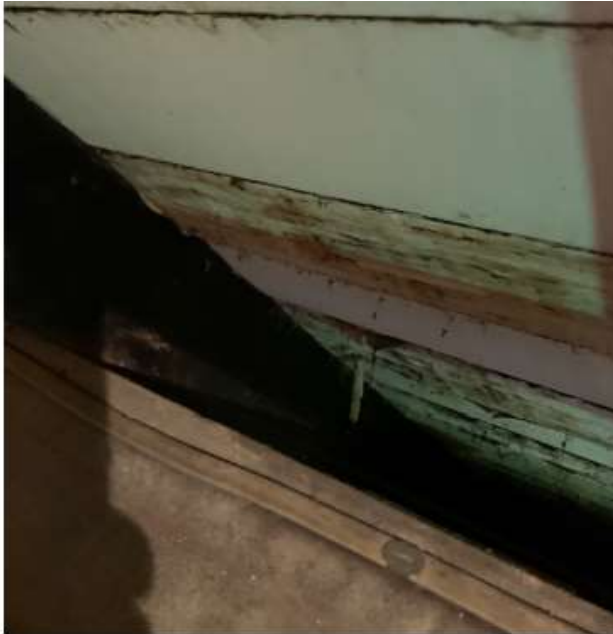
Photo showing signs of water ingress to the rear roof slope thought in line with external hole in the roof.
