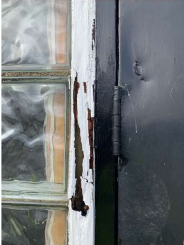
Photo showing window frame to glass brick wall in an advanced state of decay
