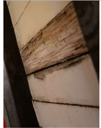
Photo showing decay of timber sarking board over the clerks office
